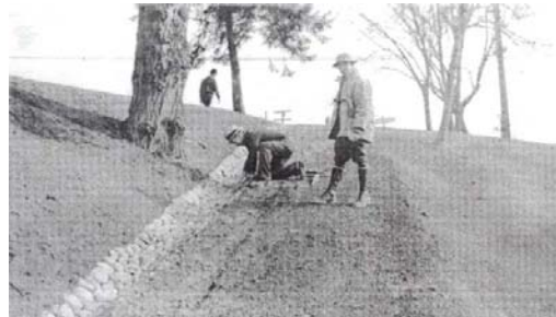
Figure 2. Forming Stone Gutter on Walk down to Shelterhouse, 1936, F. Leissler. Source: Arboretum
